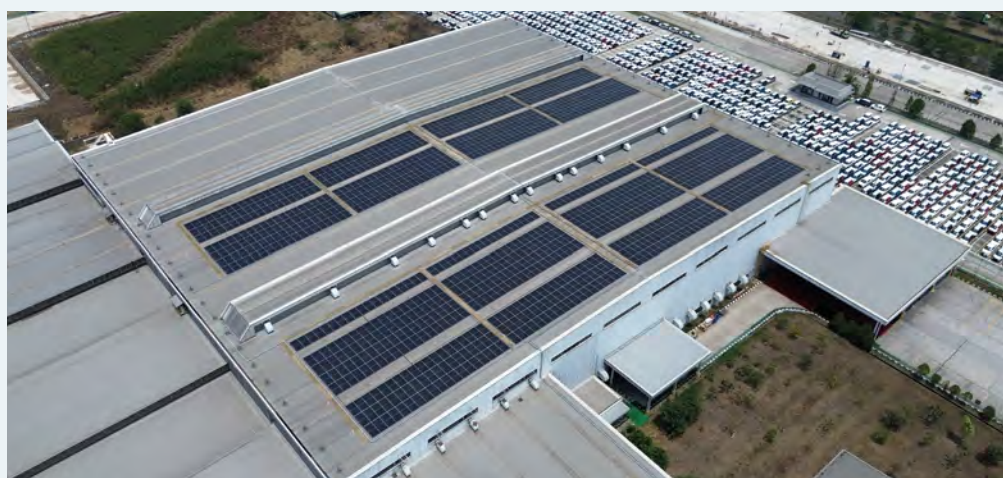
Solar panels at PT Astra Daihatsu Motor
